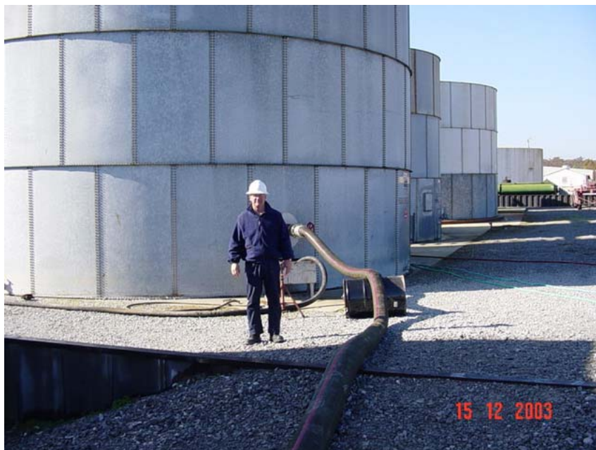
Figure 62 200 ft. 6 inch hose to waste oil tank.
