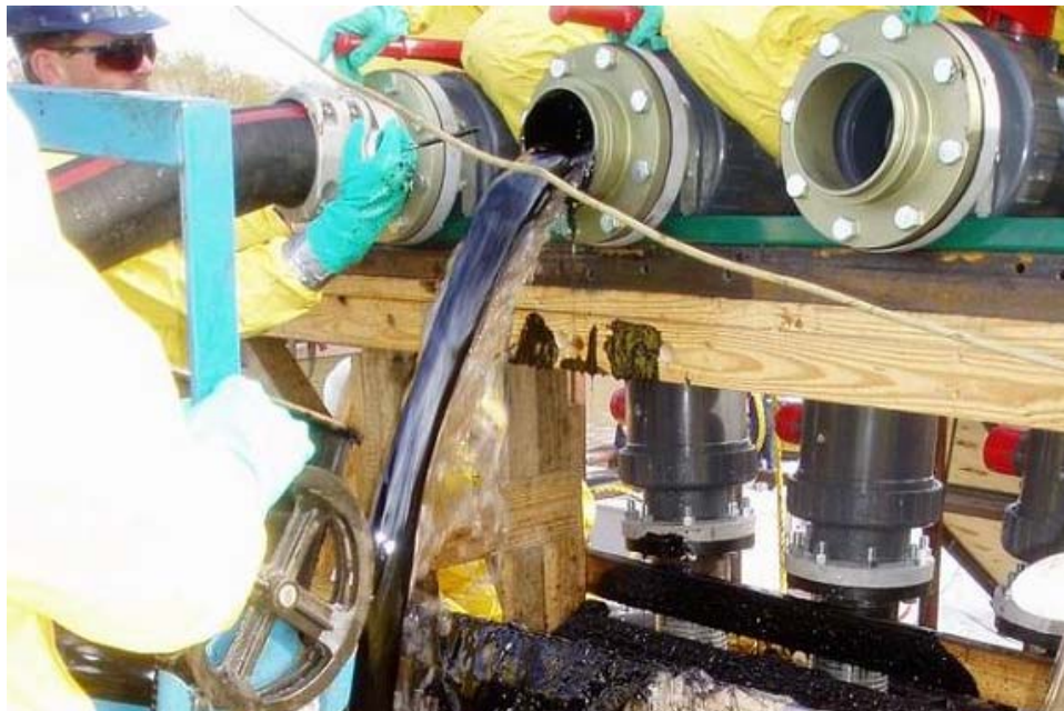
Figure 57 Oil and lube water discharge in 515 ft test with CCG GT-185 pump.
