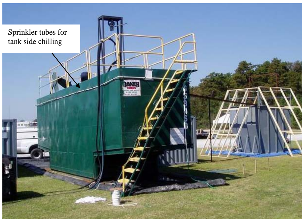
Figure 10 USCG 500 bbl Backup Tank (Baker). Note the tubes for tank side sprinkler chilling and to the right the USCG test tank.
