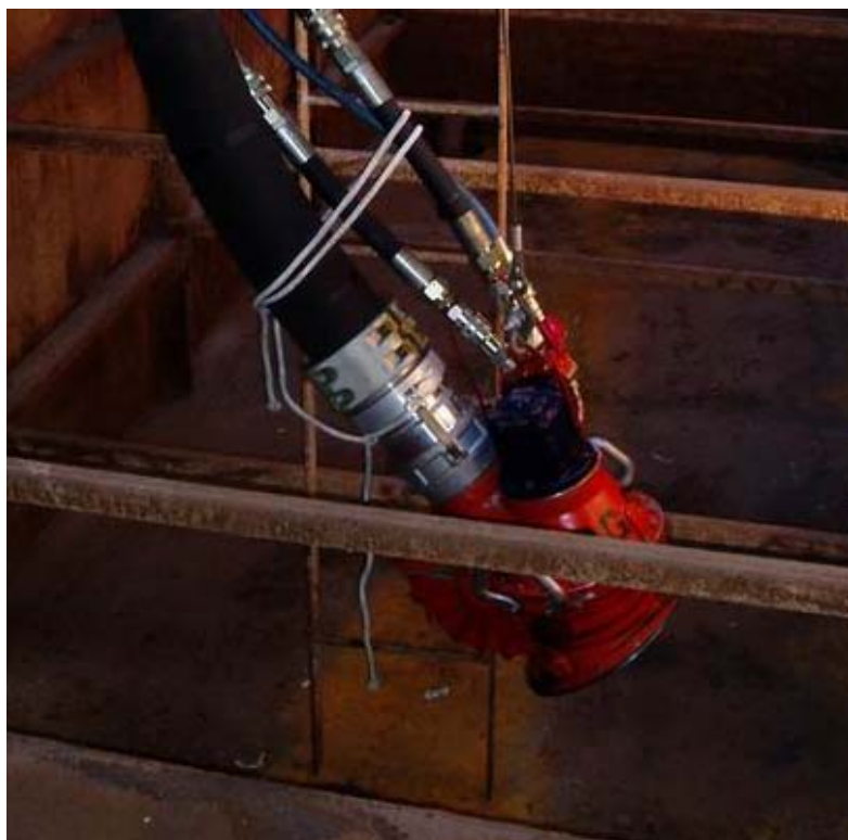
Figure 24 USCG DOP-250 Mix and Transfer Pump in Position in the USCG 500 bbl Backup Tank
