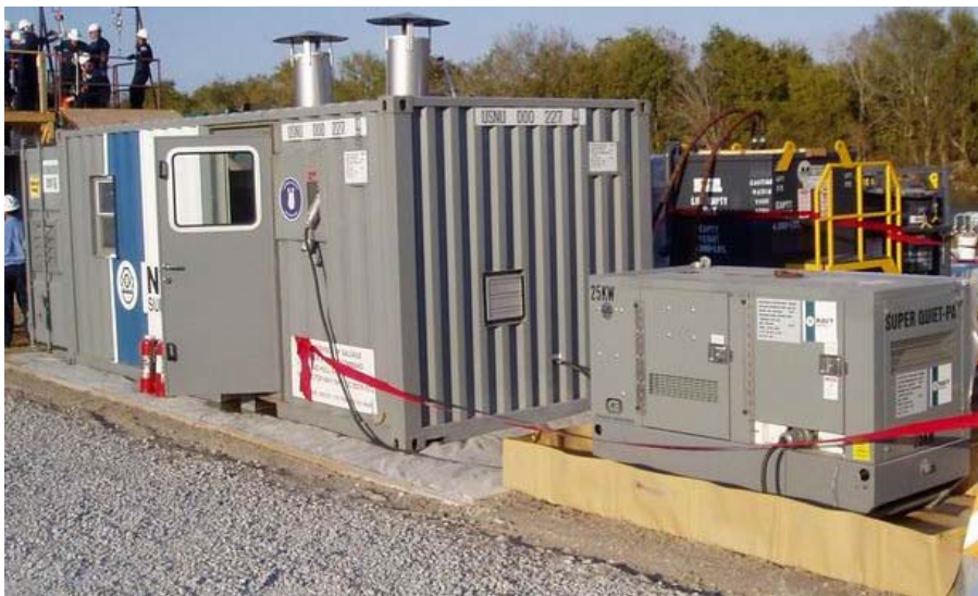
Figure 12 US Navy Containerized Clayton Boiler System with Power Pack
