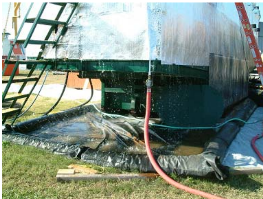
Figure 30 USCG 500 bbl Baker Backup Tank with Double Sided Reflective Bubble Plastic Insulation. Note the tank side chilling water dripping off beneath the insulation and into the containment berm where it flows to a sump for re-circulation to the chiller system.
