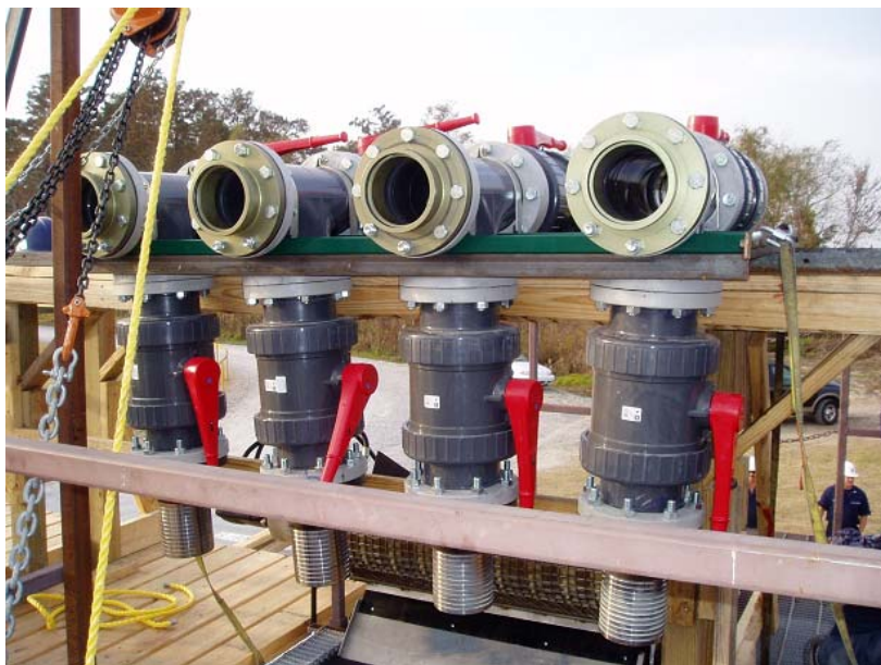
Figure 21 The Valve SHAS, here shown in position over the CCG Test Tank.
